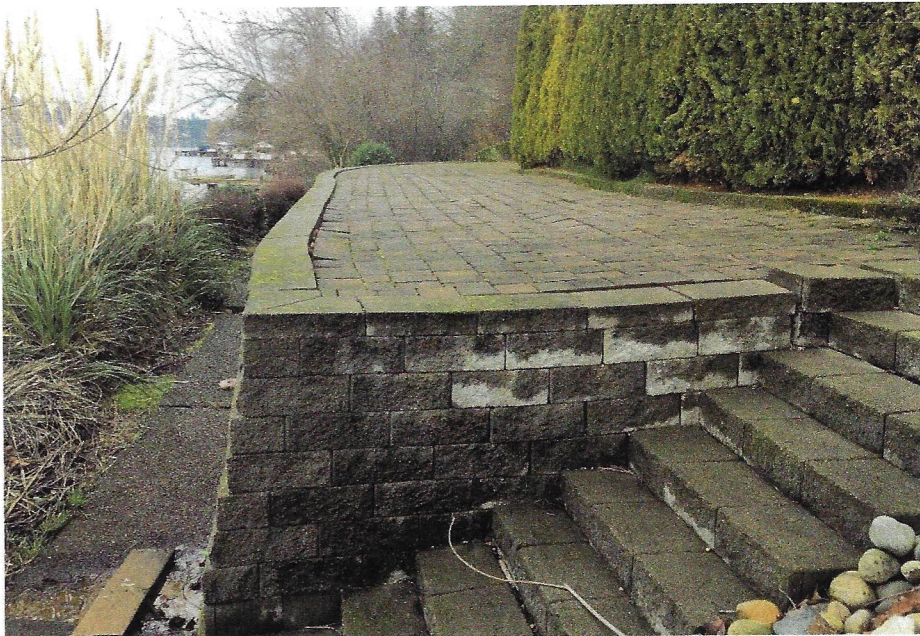
(8) Patio 2 Pavers. Looking North. Note curved CMU wall top, and pavers that have settled relative to the wall. Gaps between pavers indicate lateral movement toward the lake.
