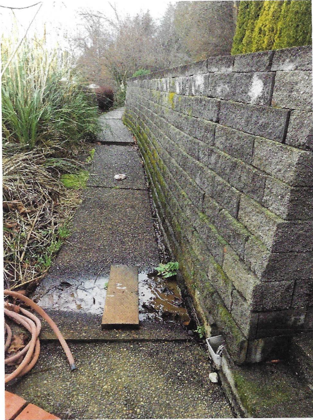
(7) Patio 2 CMU Wall. Looking North. Note apparent sidewalk settlement close to the photographer, curved wall face, and groundwater seepage. In addition to visible seepage in the foreground, the moss along the bottom tiers of the wall indicate moisture for seepage.
