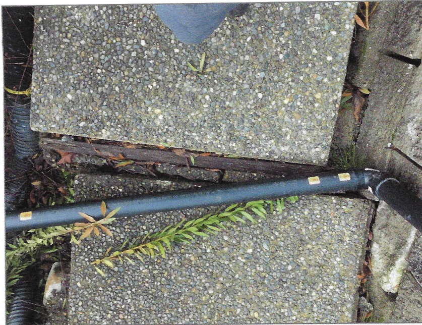
(3) Closeup of 7701 Sidewalk. January 5, 2019. The top of the photograph is towards the lake (west). Note the temporary sewer line. The downhill panel is offset 6 inches to the south and about 5 3 / 4 inches to the west.
