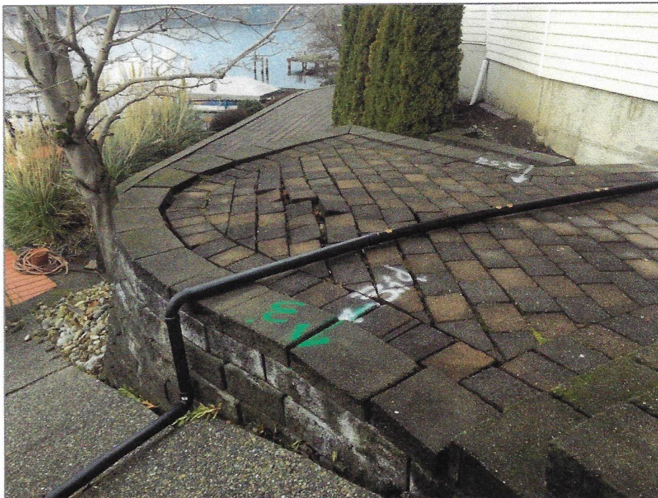
(6) Patio 1 Pavers. Looking west. Note the settlement relative to the wall and the openings between the pavers caused by lateral movement.
